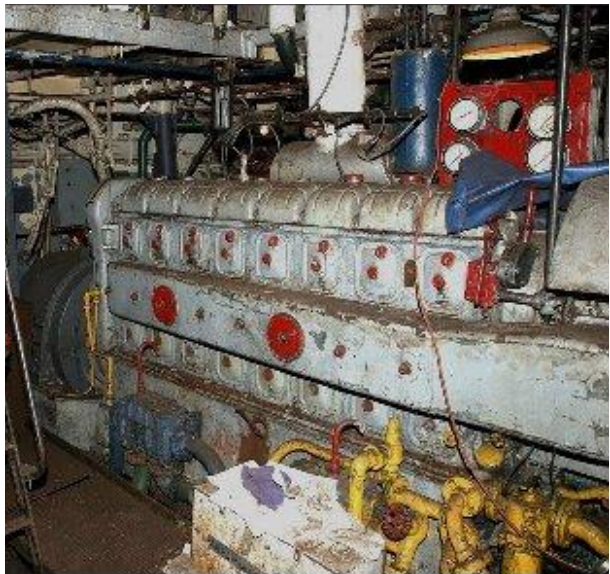
The generator has had a rough life.
