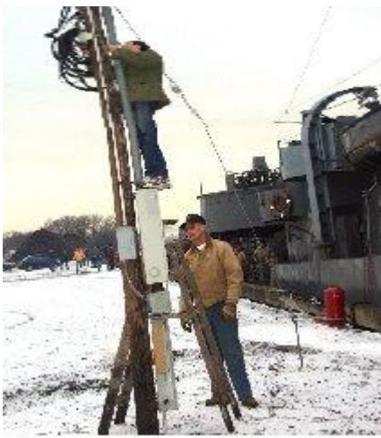
Barry and Benner hooking up the shore power.
