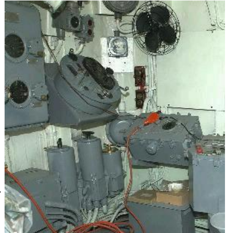
Michigan Dick Walker's restored fire control room.
