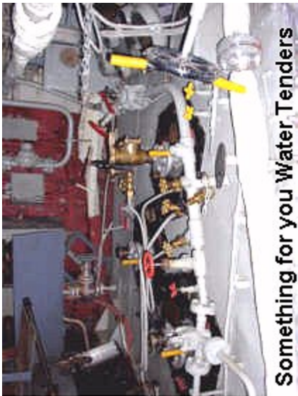
Boiler Face in B1, APD 128
