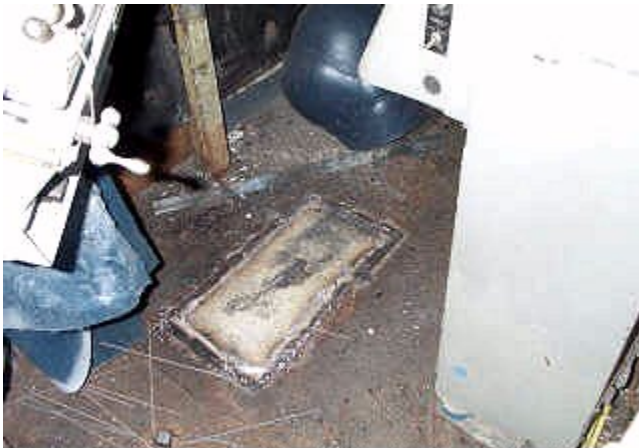
One of Several New Patches in the Pilothouse Overhead
