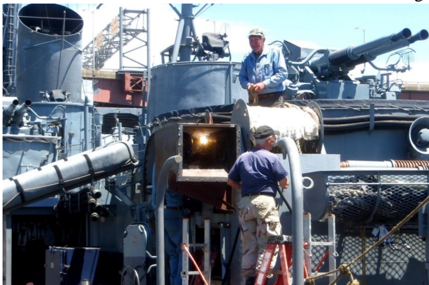
The big project for the shipfitters has been the aft supply vent intake fabrication.
