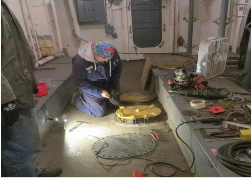
Doug Tanner and his shipfitters repaired all the wasted and damaged metal in the aft berthing compartment.
