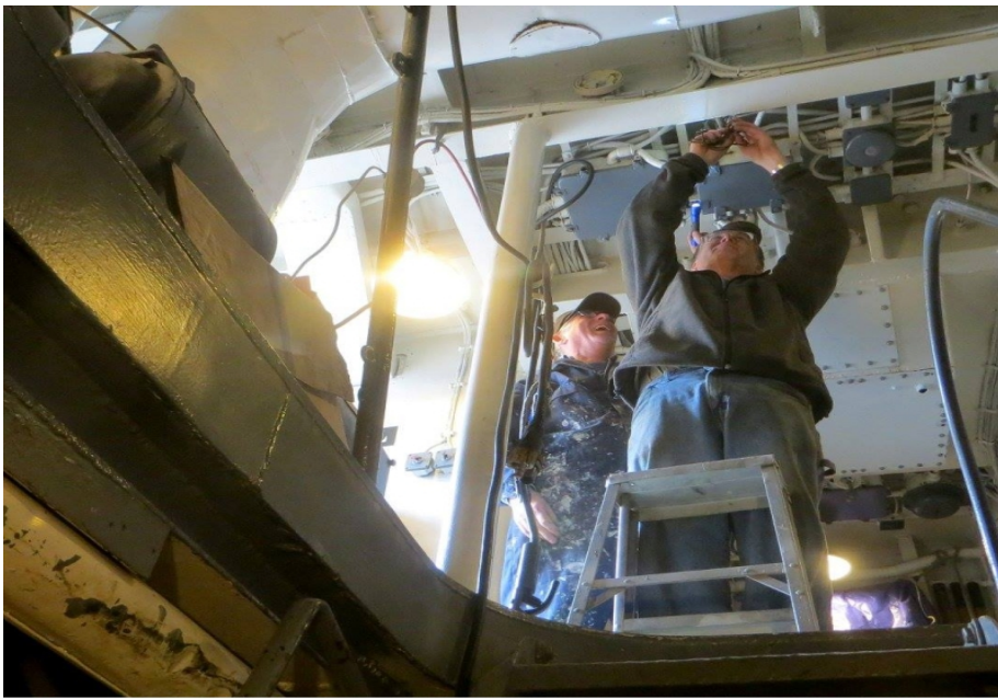
Gary Sheedy and Barry Witte tidied up a lot of the cable runs prior to repainting.
