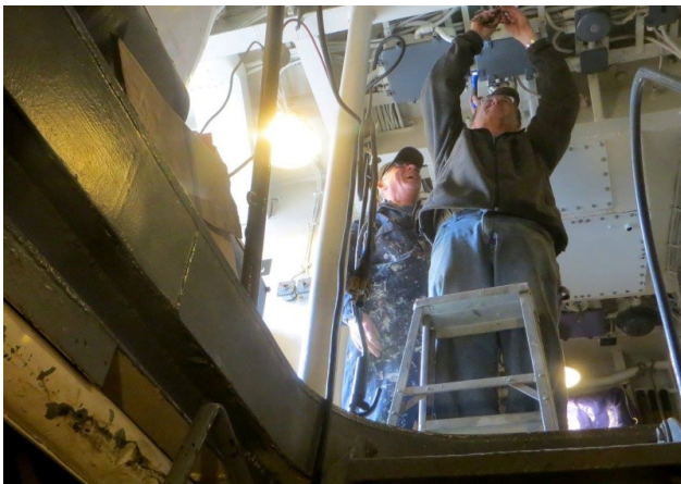
Gary Sheedy and Barry Witte tidied up a lot of the cable runs prior to repainting.
