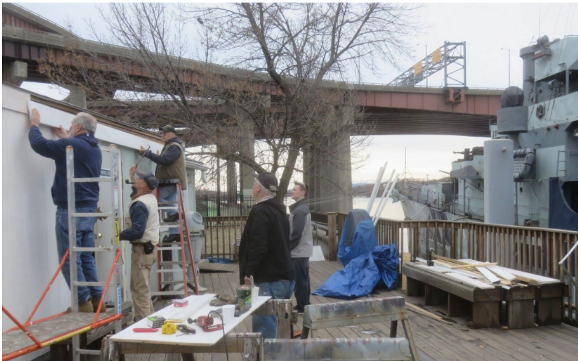
The crew took advantage of the few warm days to continue work on the trailer rehab.
