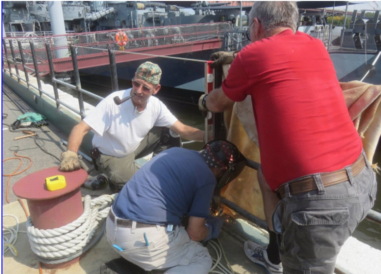
The continuing project for the shipfitters has been the seawall safety rail.
