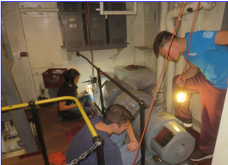
RPI NROTC Midshipmen installing the inspection covers on the B-3 motor generator.
