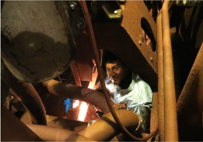
Preparation for the fleet. It takes an agile Sailor to fit under the fire and flushing pump.
