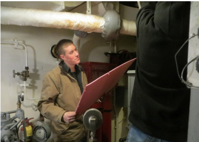
Jim Lenden and Barry Witte closing up the B-3 vent ducts for the winter.
