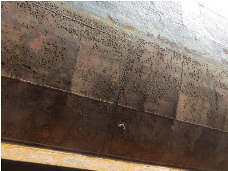
Pitting revealed in drydock after sandblasting.
