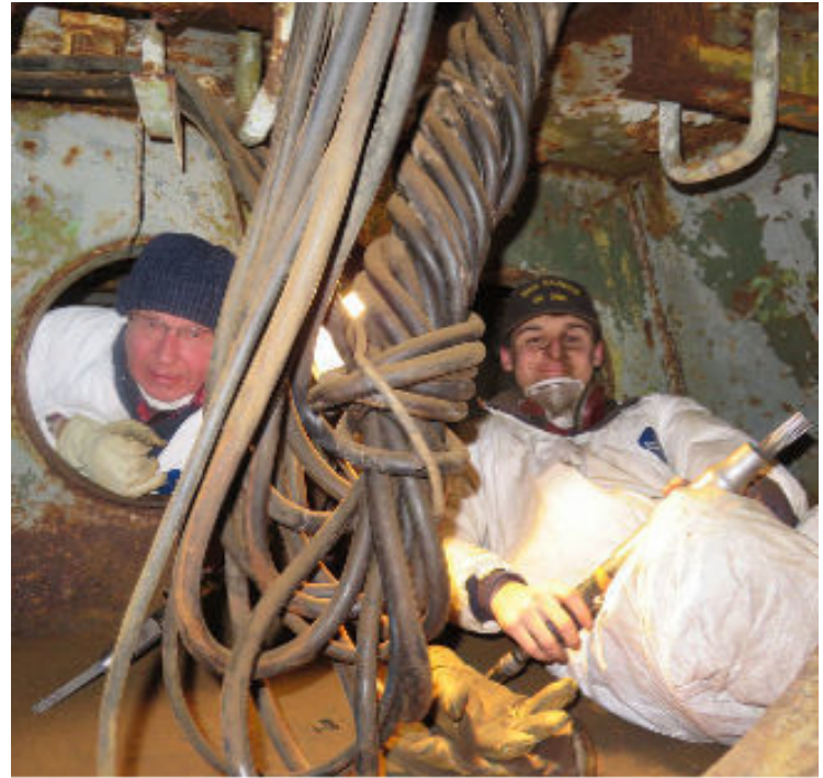
More inside work as Ron Mazure and Thomas Scian scaled under the gun three tub in preparation for welding.
