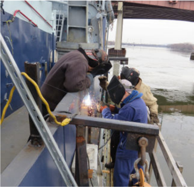
Early in the month we finally finished the welding on the davit pedestal project, but painting will have to wait for spring.
