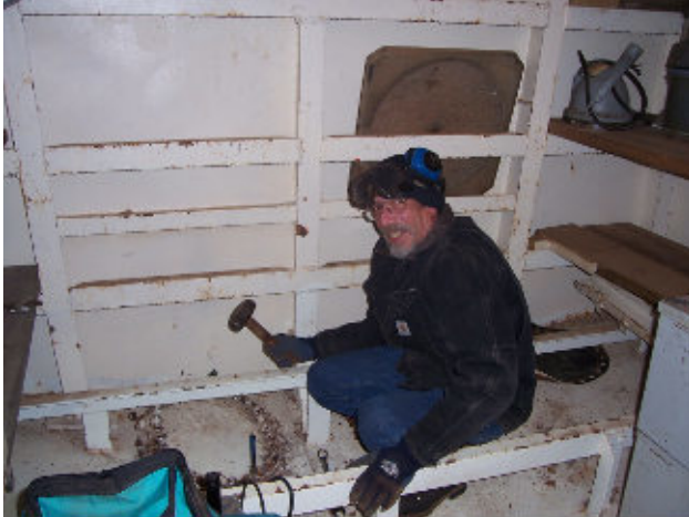
It was about ten degrees in the magazine when Bill Wetterau was working on one of the last manhole covers.
