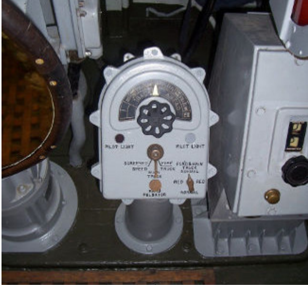
The restored speed light controller in the pilothouse.
