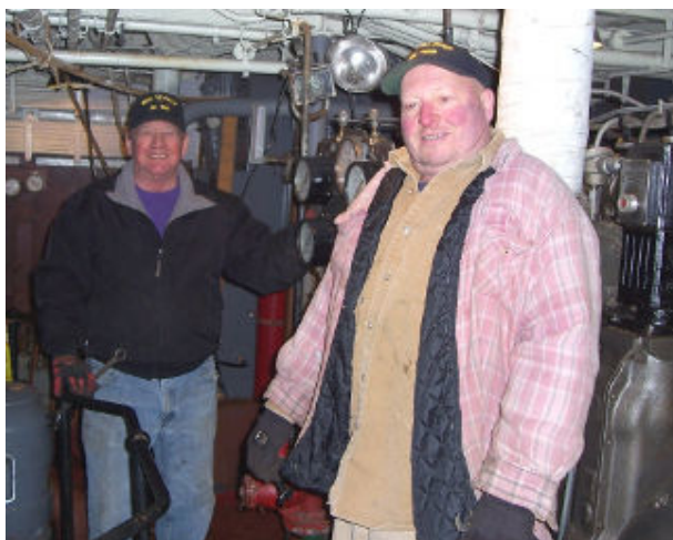
Ken Myrick and Mike Dingmon work to get the emergency diesel back on line.
