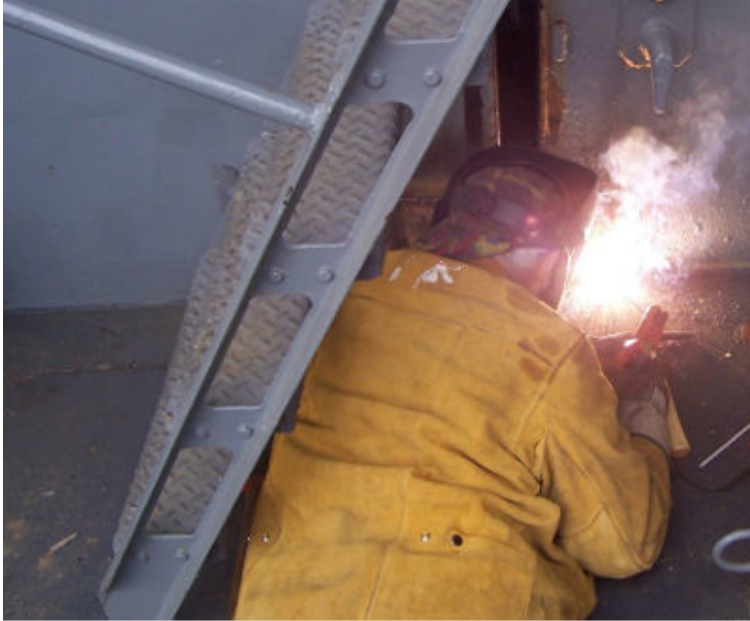
"Super Dave" Mardon welding up the starboard base of the expansion joint.
