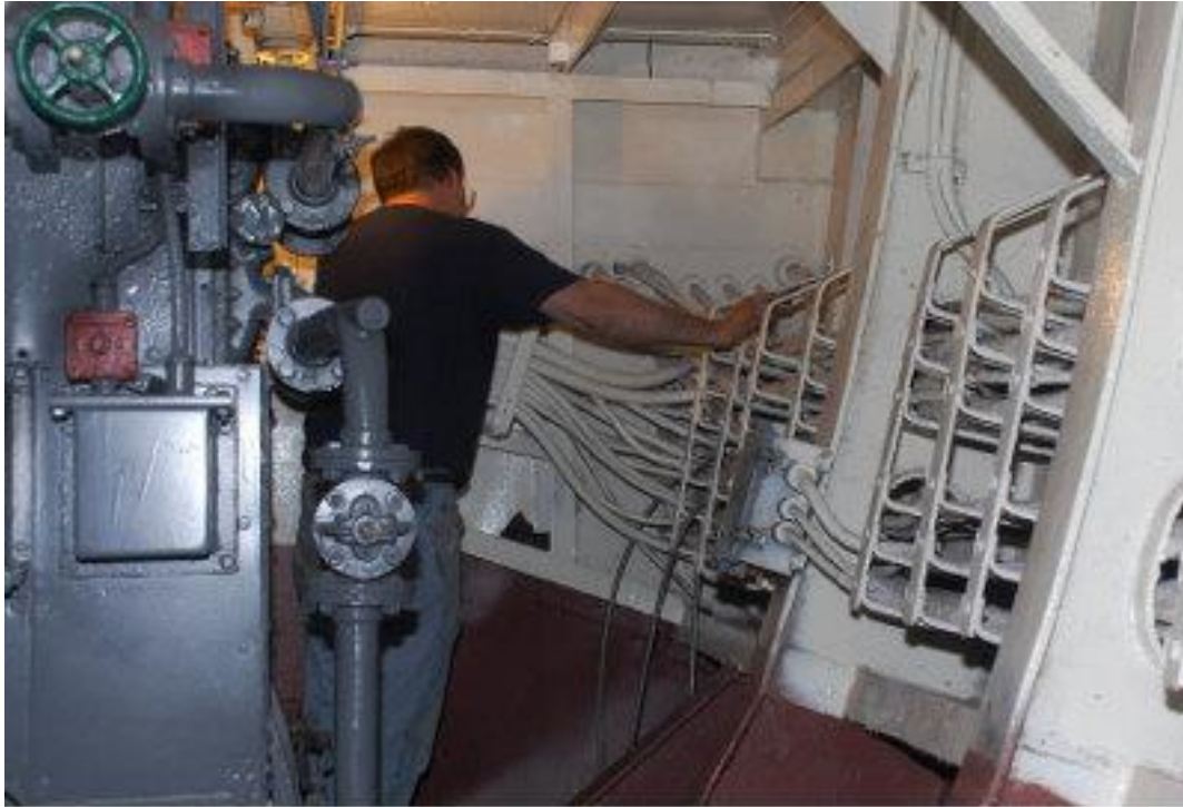
The restoration work continues as Barry Witte traces electrical cable in the lower level of B-4.
