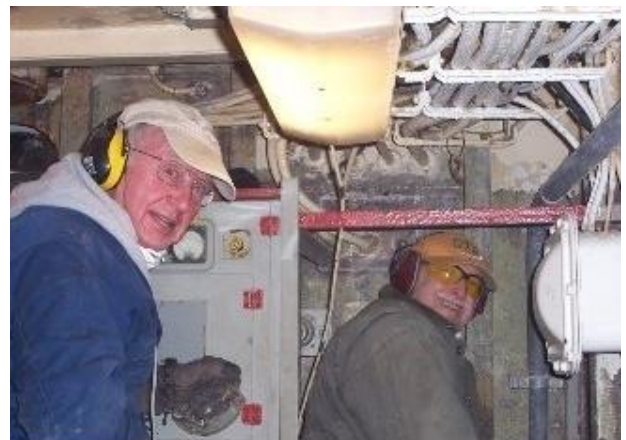
Ron Mazure and Don Miller chip out the ET shop below the messdecks.
