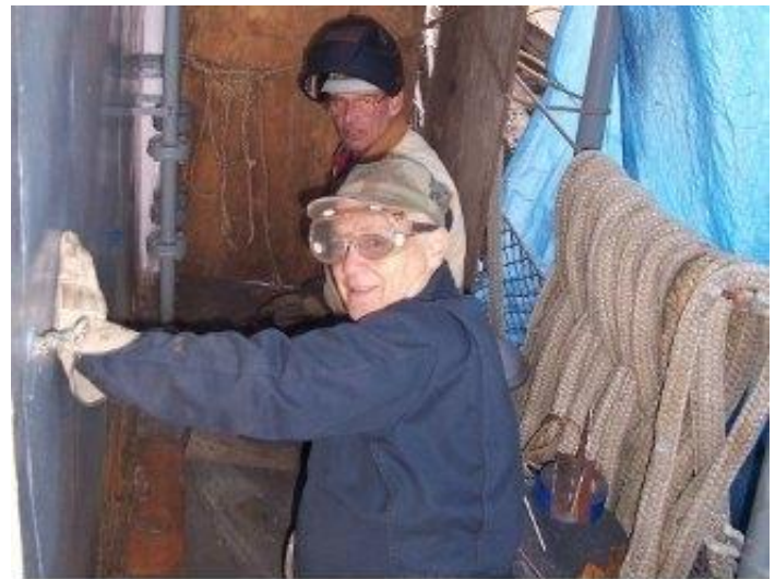
Tim Benner and Dave Mardon replacing wasted steel in the starboard deckhouse.
