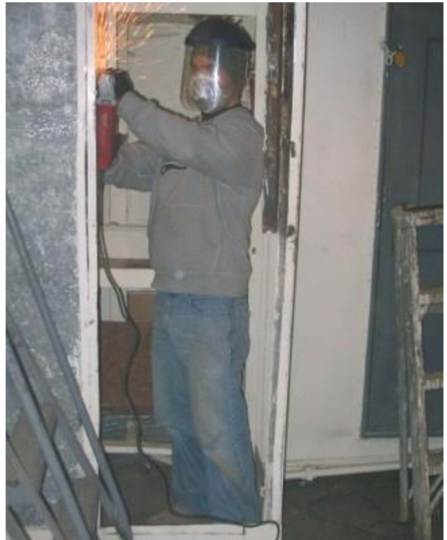
Work on the messdecks storeroom. Mike Forstner grinds to fit a new bulkhead panel,
