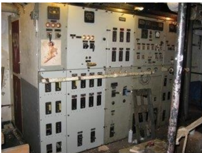
The aft main electrical distribution panel in B-3 before...
