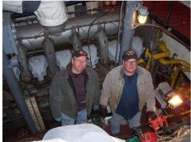
Gary Lubrano and Mike Dingmon working on the restoration of number four main engine.
