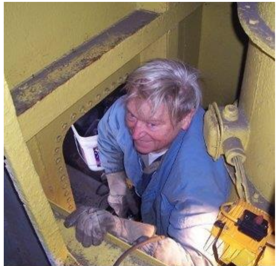
...the ones that stayed behind are carrying the load. Here Gene Jackey crams himself into a fan to weld the repair steel plate.
