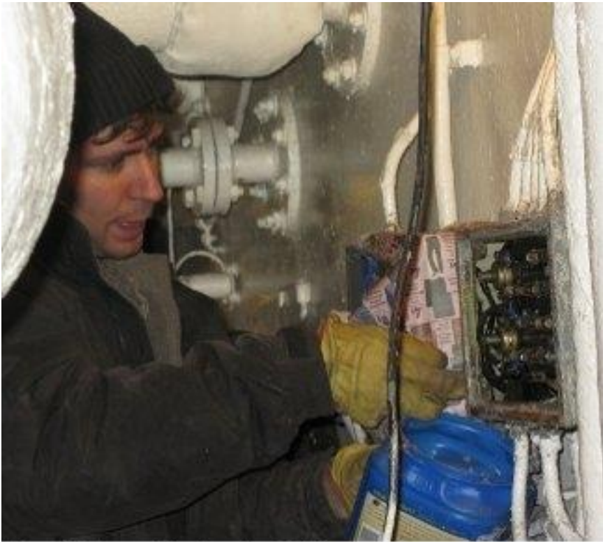
Paul Guarnieri refurbishes the paint job on a switch box on the upper level of B3...
