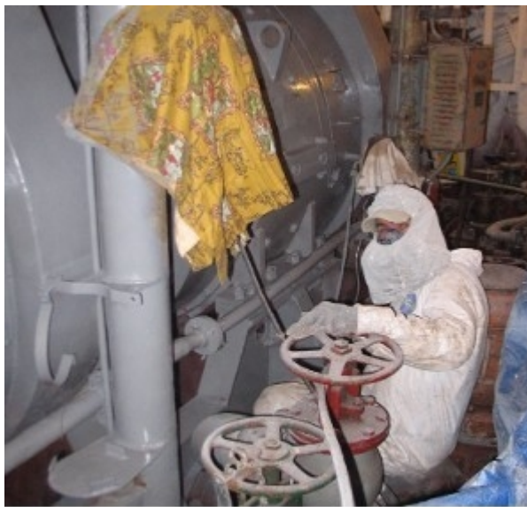
... and the main propulsion motors in B-4.
