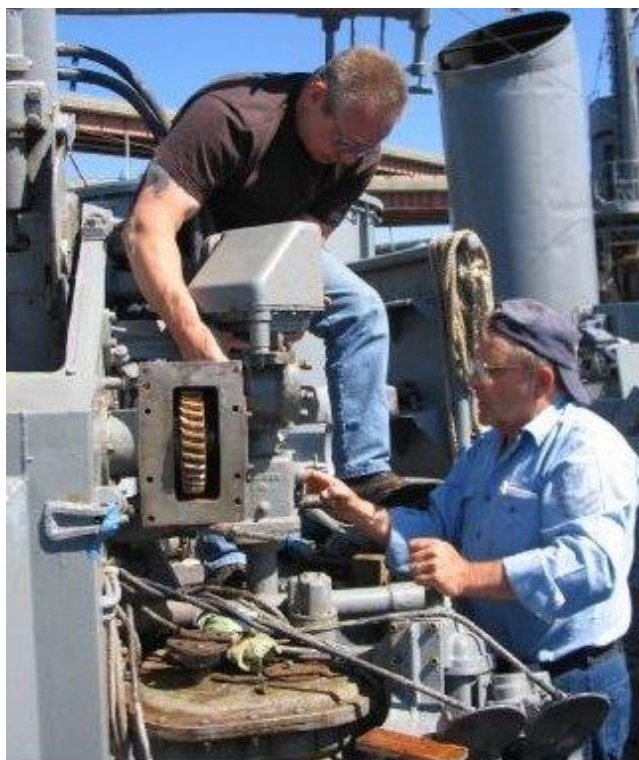
After waiting a couple weeks for the replacement gears, Gary and Gus spend an afternoon putting the gun back together.
