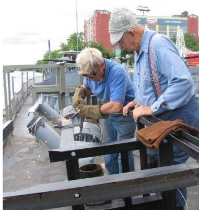
Gene Jackey and Clark Farnsworth put together one of the replacement depth charge racks.
