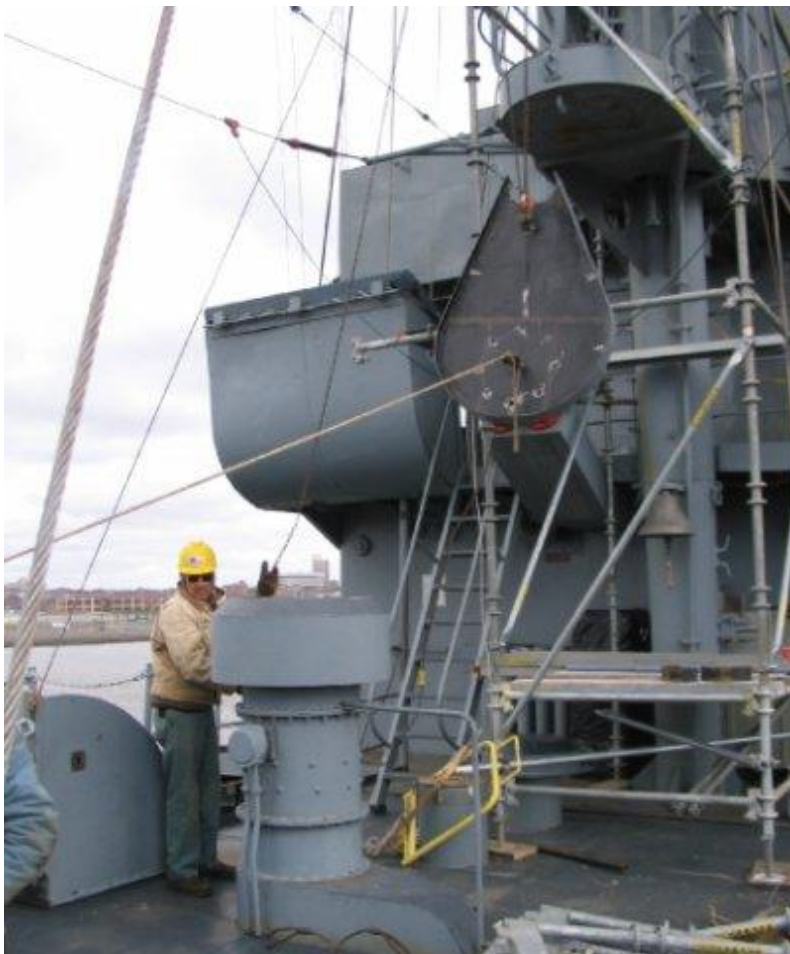
Tim benner uses a chain fall to lift the SL radar platform up the mast.
