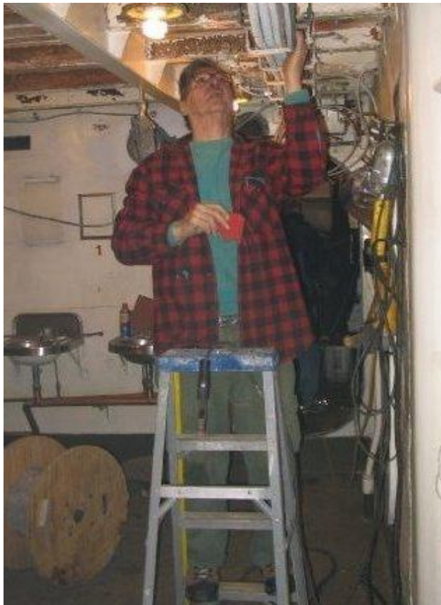
Joe Breyer prepares to weld a new cable bracket to the washroom overhead.
