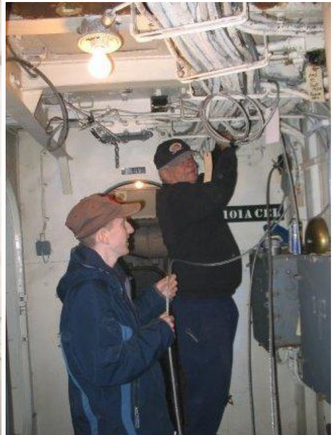
Further aft, new cable goes in to replace worn and corroded cable.
