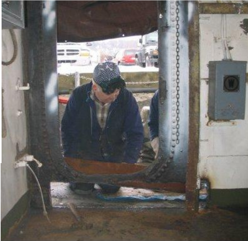
Doug Tanner checks the fit of the aft passageway starboard side patch.
