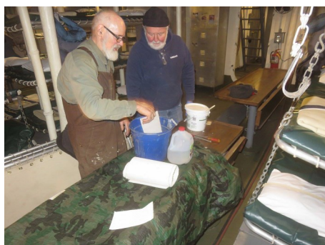
Tommy Moore teaching Rich Mouzakes the fine art of fiberglass insulation repair.
