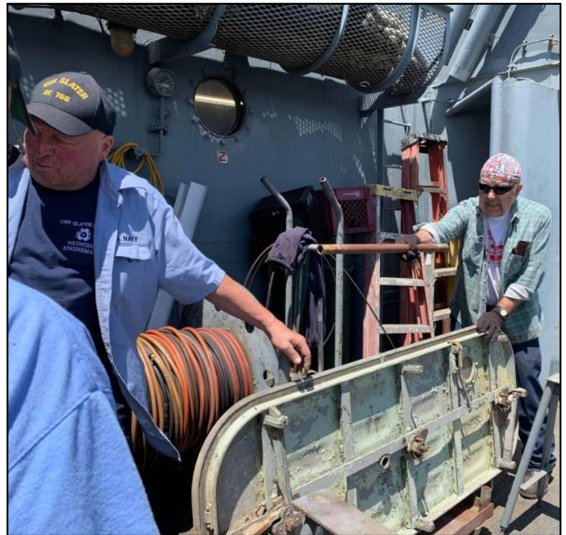
Mike and Doug move the watertight door to the workbench for repairs.
