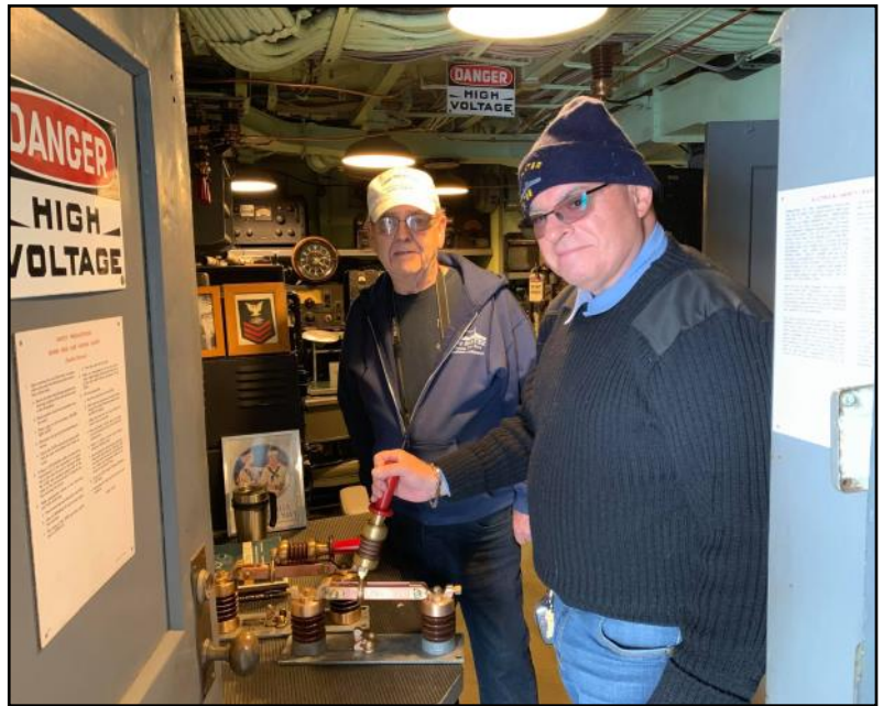
George and Chuck check out the disconnects George made.
