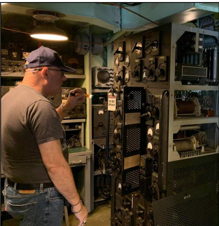
Chuck is studying the complexities of the TBL transmitter in the radio room.
