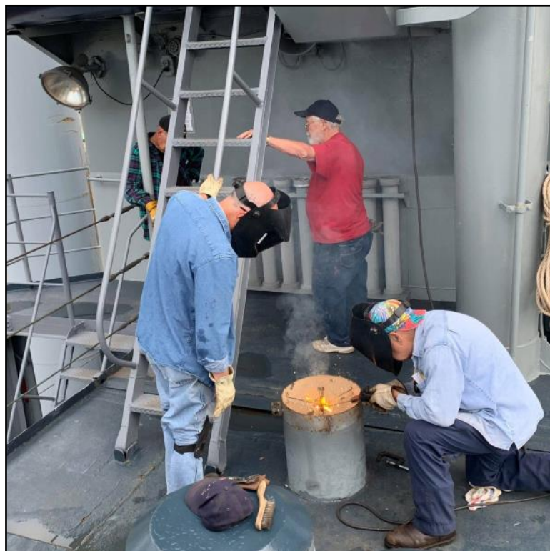
Gary drafted the whole crew to help him out with the galley supply vent.
