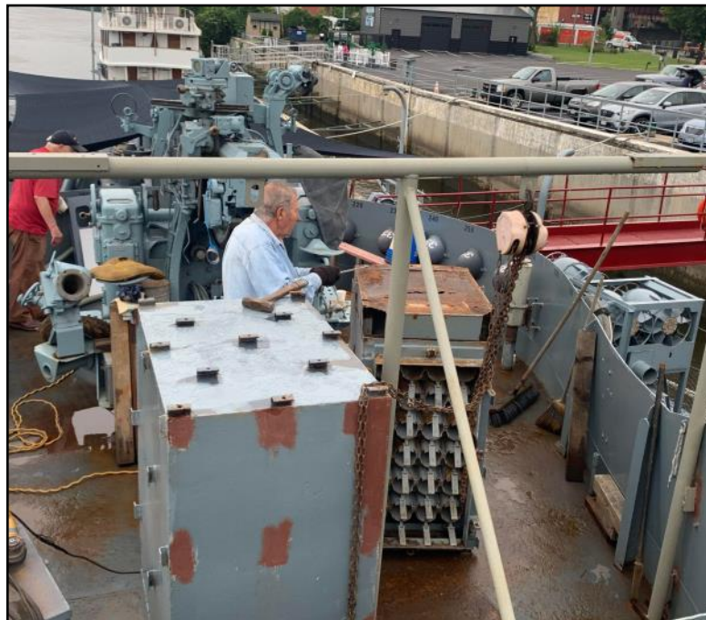
Danny completed the repairs to the starboard ammo locker, and is now working on the port locker.
