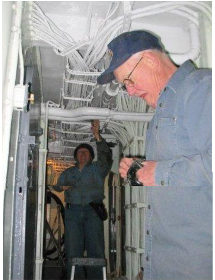
Gene Jackey and Don Shattuck replacing restored light fixtures in the freshly painted midship passageway.
