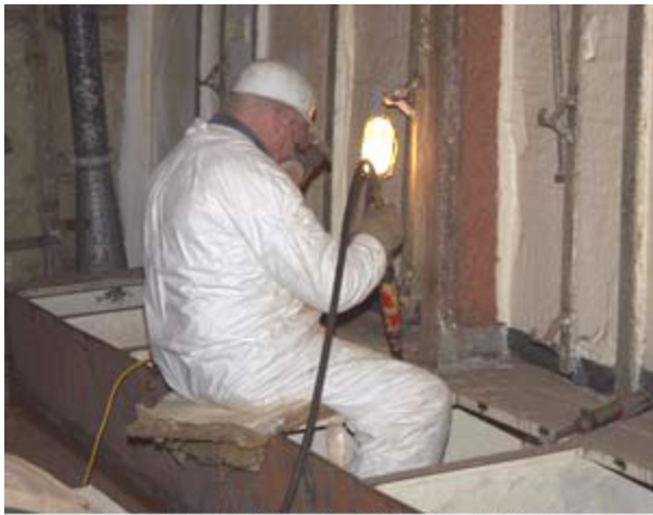
Ed Whitbeck Chipping Paint
