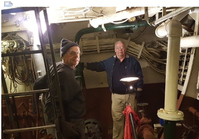
Larry Williams and Karl Herchenroder at work in the aft engine room.
