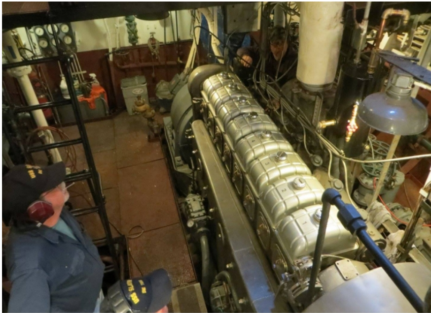
The engineers did a successful test run of the B-3 ship's service generator.
