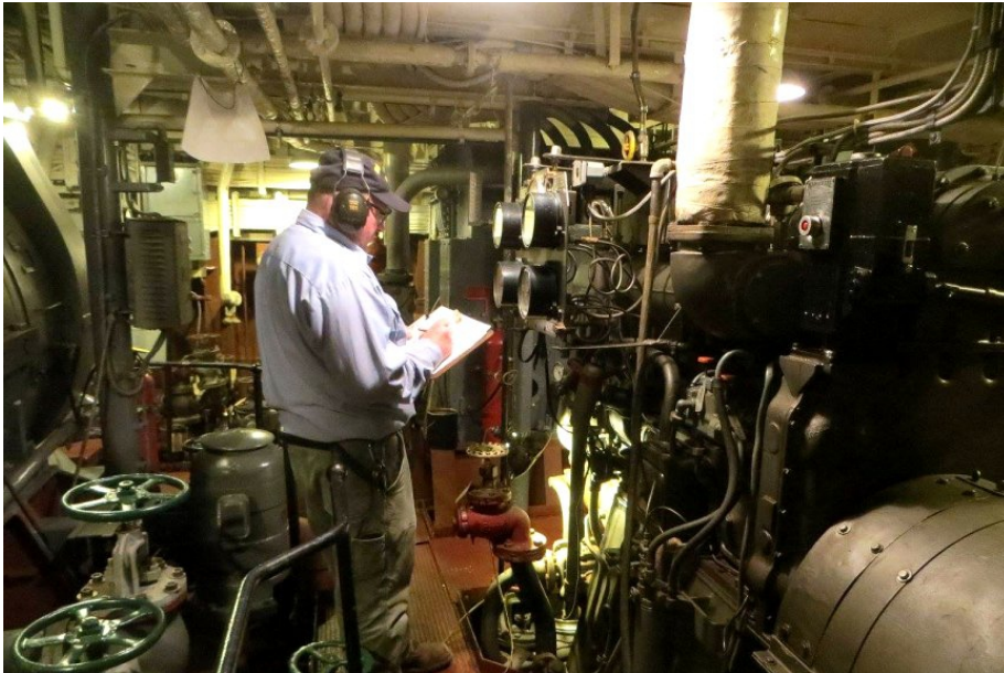
Mike Dingmon takes temperature readings during a test run of the emergency diesel generator.
