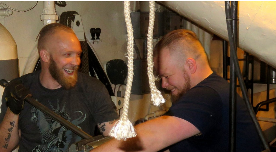
Vets Shaun and Pat Sutton from College of St. Rose working on the firemain.
