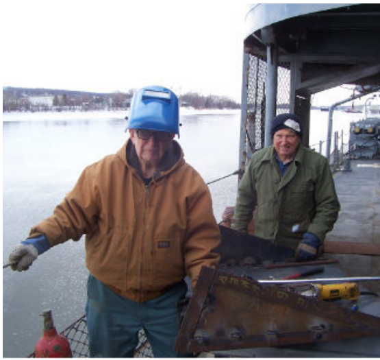
Clark Farnsworth and Gene Jackey fabricating the new 40mm spent case chute.
