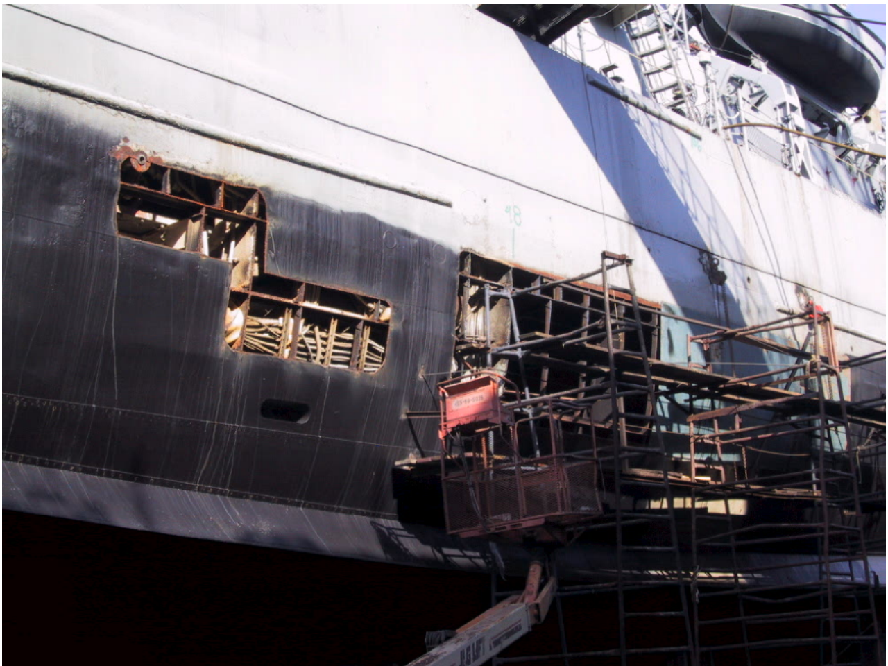
This photo off USS EDSON shows the type of repair we hope to do on SLATER.
