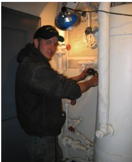
The mess deck water heater gets valve handles courtesy of Will Tryon.
