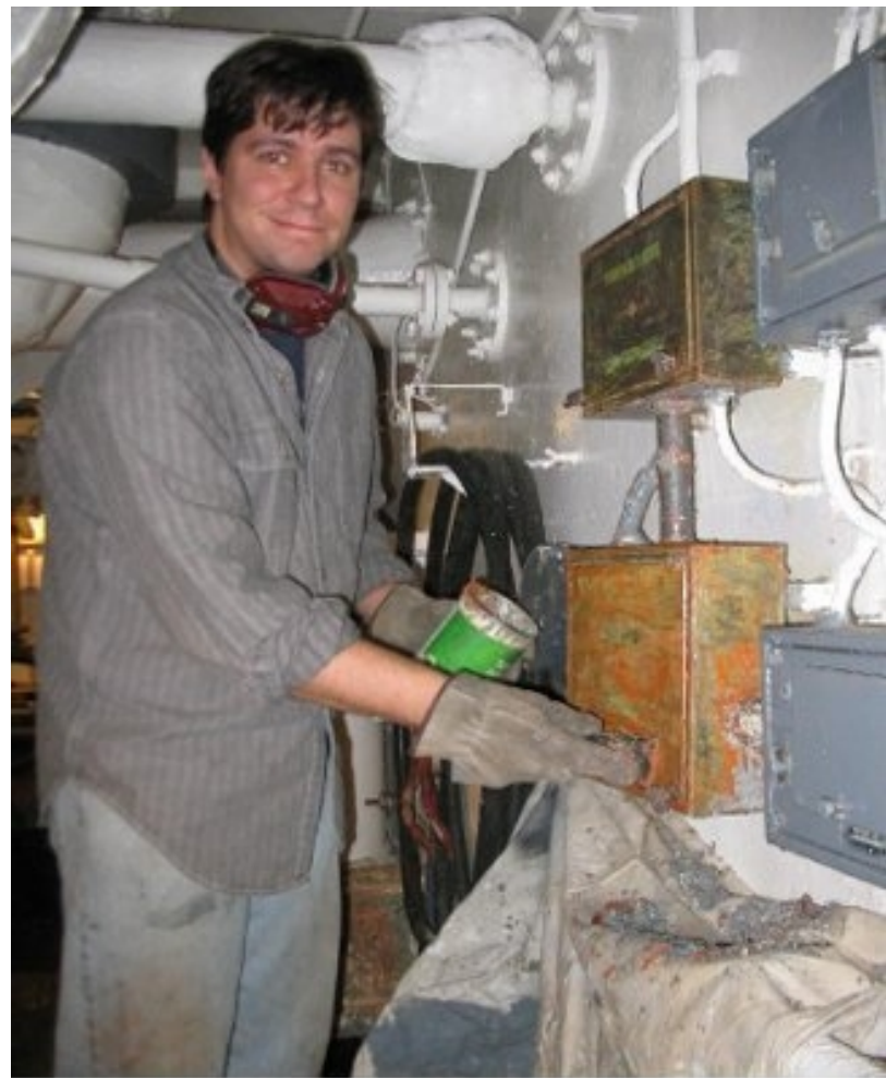
...by the boys in B-3, doing detail work on the electrical box restoration.
