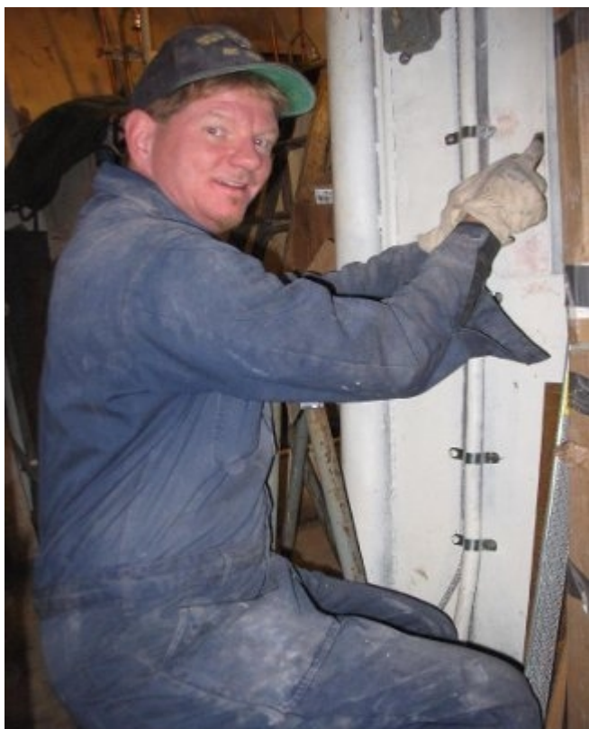
Former USS IOWA machinist mate Mike McEnteggart applying bondo in the forward head.
