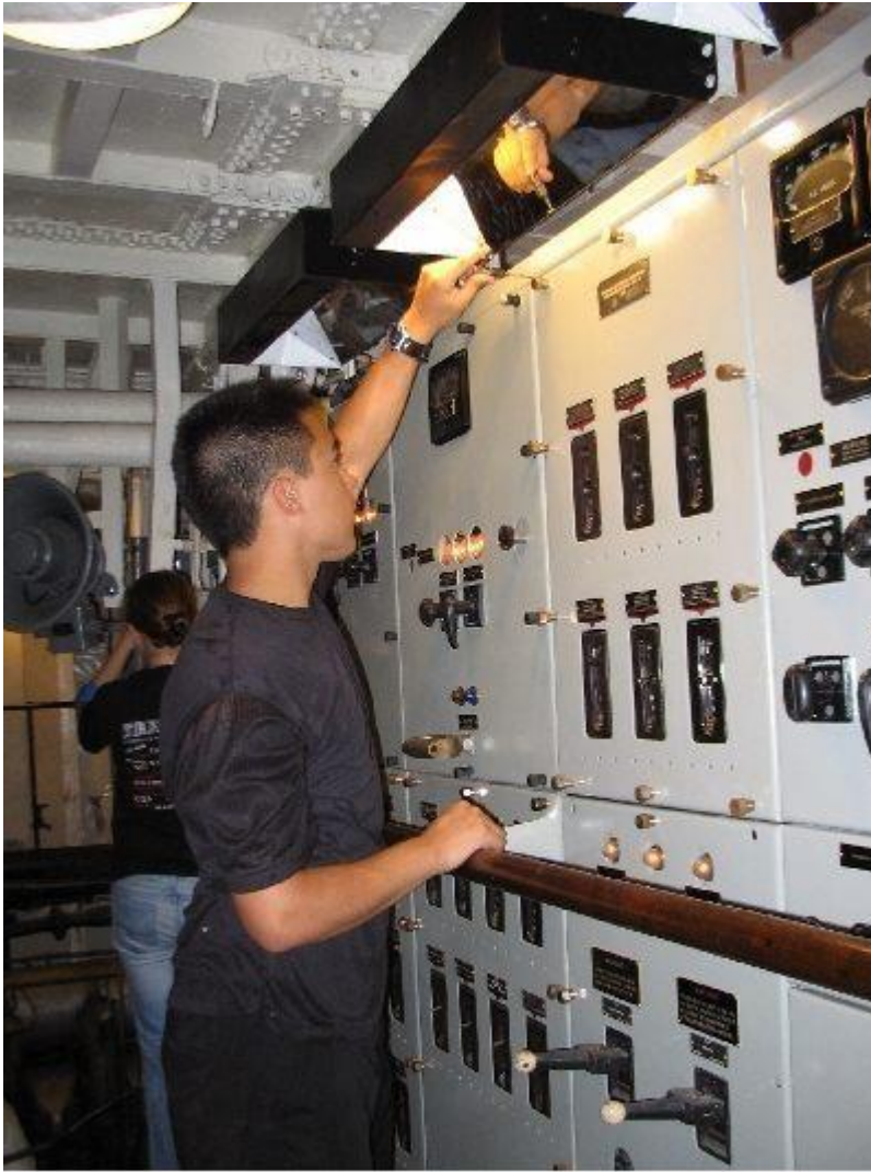
RPI Midshipmen assisting with the restoration of the electrical distribution board in B-3.
