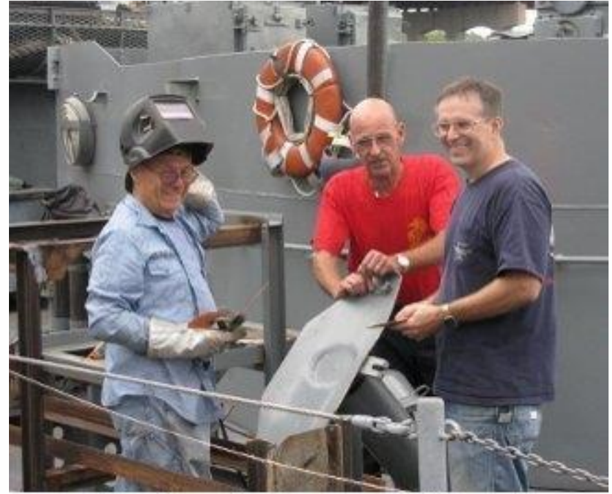
Dave Mardon, Tim Benner and Barry Witte have been making progress on the number six roller loader fabrication .
