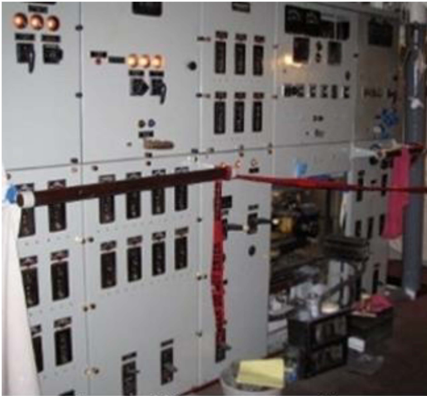
Barry Witte and his crew are making progress on the B-3 switchboard.
