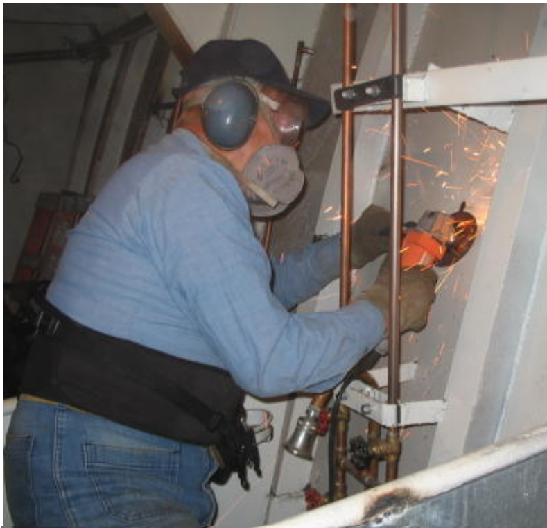
Gene Jackey hard at work grinding off old stubs in the forward head.
