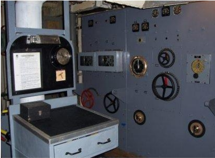
Progress in the aft motor room. The aft electrical board being restored by George Gollas and Barry Witte.
