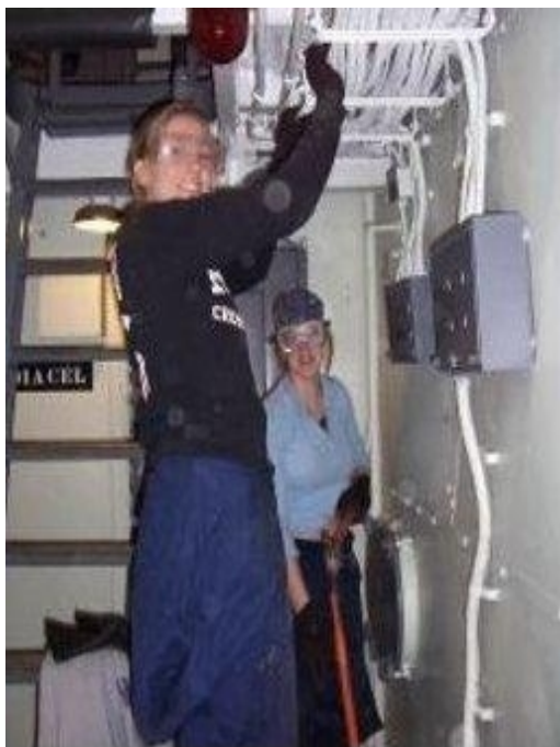
Remember the phrase, "This man's Navy?" Those days are over. Midshipmen Kelly Gardner and Shayna Palesch pulling armored cable outside the radio room.
