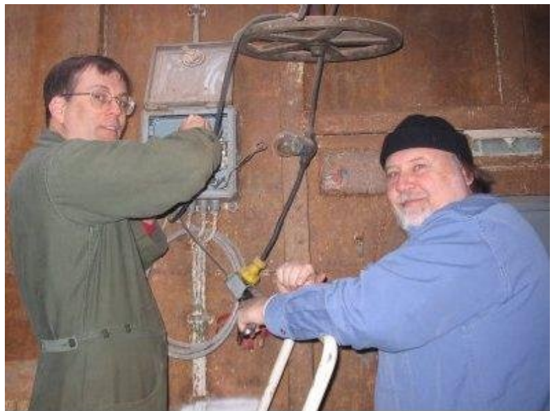
Barry Witte and George Gollas are working on replacing a switchbox in the forward passageway. (When the engineers give them leave from B4.)
