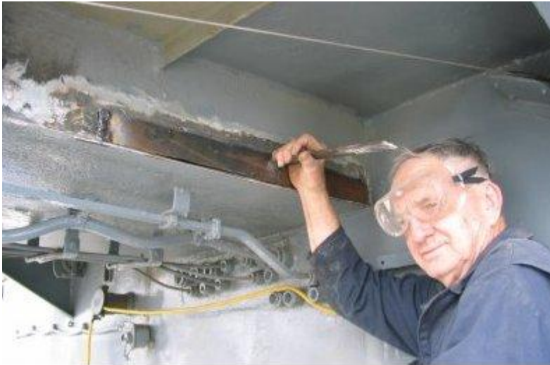
Jim Ray helping the team that patched the RDF platform on the bridge.
