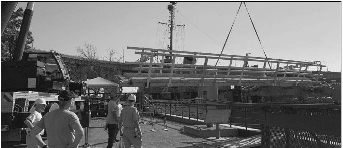
Three D Rigging helped us out with a crane to move the temporary gangway into place.
