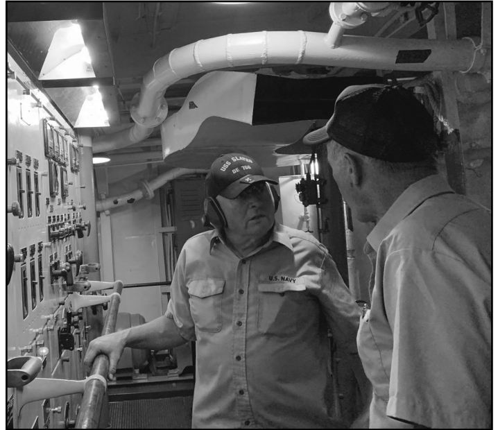
Mike and Gary making sure the generator stays running on our shipyard trek., while it was 103 degrees in the engineering spaces.
