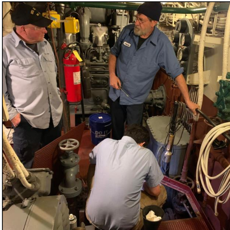
The engineers have winterized the diesels. With your support they will be working on bilge preservation throughout the winter.
