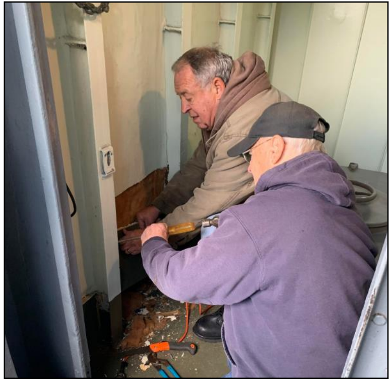
Walt and Super Dave and the rest of the shipfitters will continue to work all winter long.
