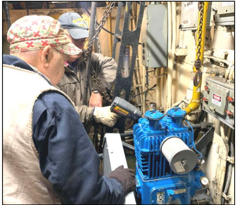
Doug and his crew completed overhaul and installation of the Quincy Air Compressor.
