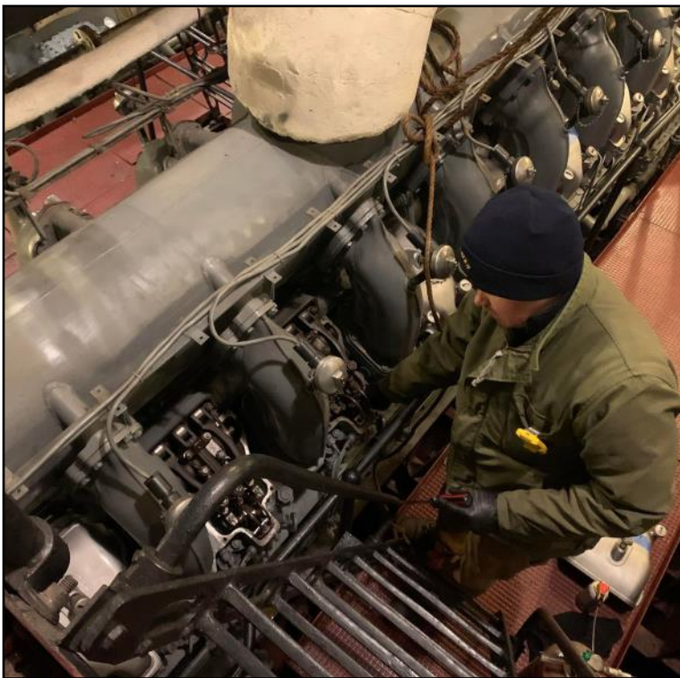
James continues his exploration into the condition of main engine number four.
