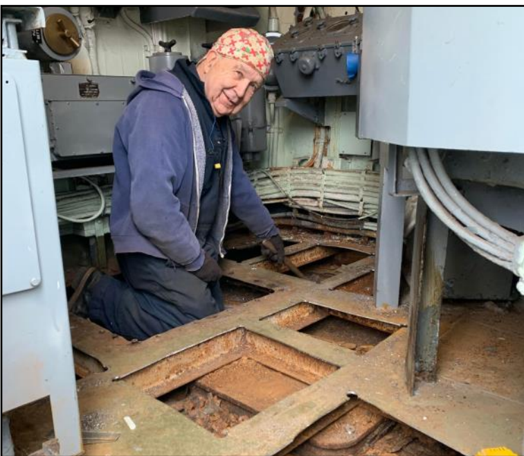
Cutting away the false deck in the radar room. Wherever Doug goes, corrosion seems to follow.
